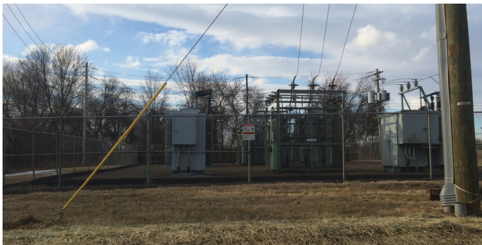
PECO Audubon substation, near PJM headquarters. © RTO Insider
